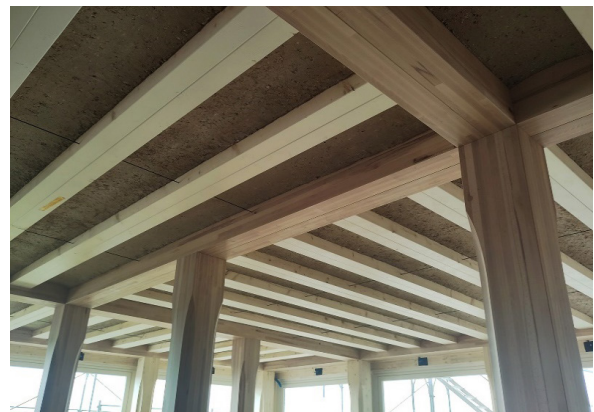
Ceiling in project HORTUS by Herzog & de Meuron Architects / ZPF Ingenieure. Source: authors.
