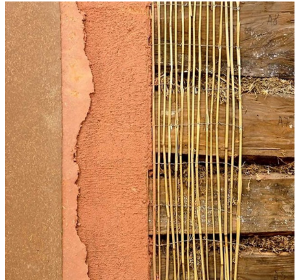
04 Layers of clay plaster system on a log wall. Source: Saviukumaja OÜ.
