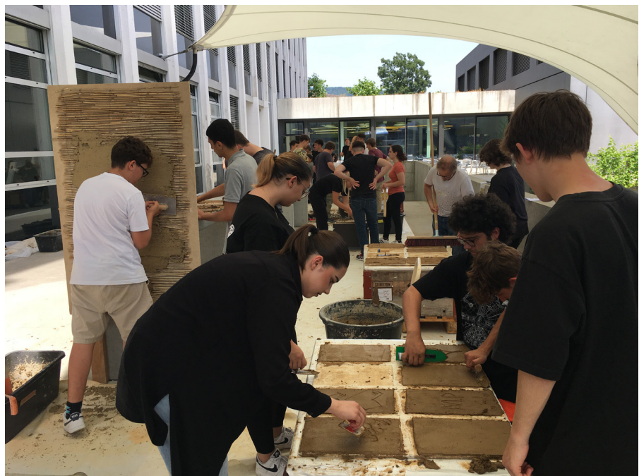
02 Clay plaster: first-hand experience of the material and building methods. A project day at Aarau Vocational School, 2023
